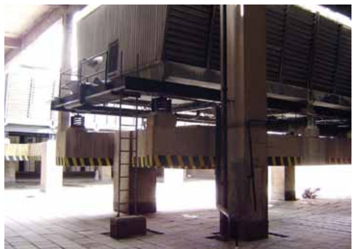
Figure 2: The existing two-story space at the 48 th floor where the original cooling tower was placed. This tower and supporting structure were demolished to allow for the new 49 th floor.
