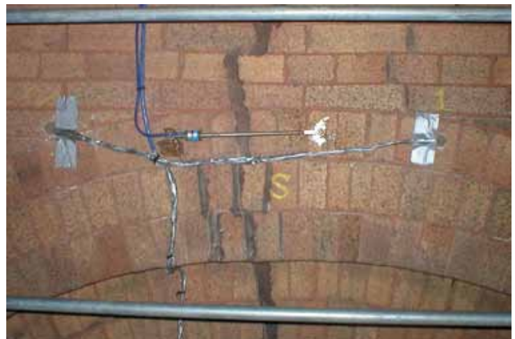
Figure 3: Crackmeter and Thermocouple Wiring Above Floor 10 Arch.
