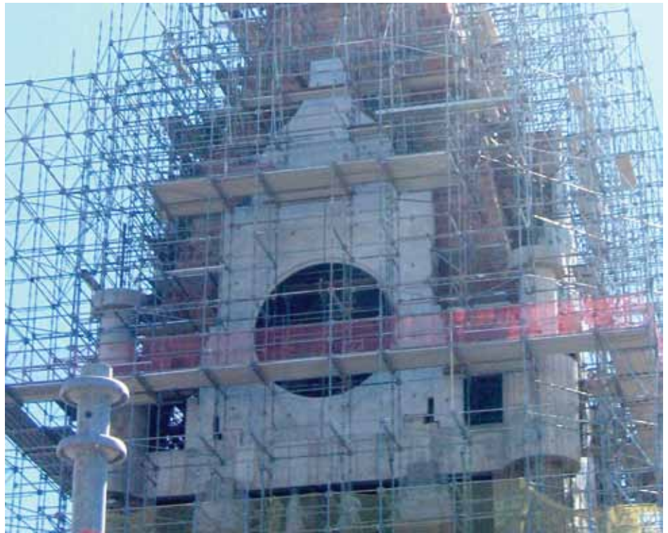
Figure 5: View of the ring beam, corner turrets, and clock gable precast backup during construction.
