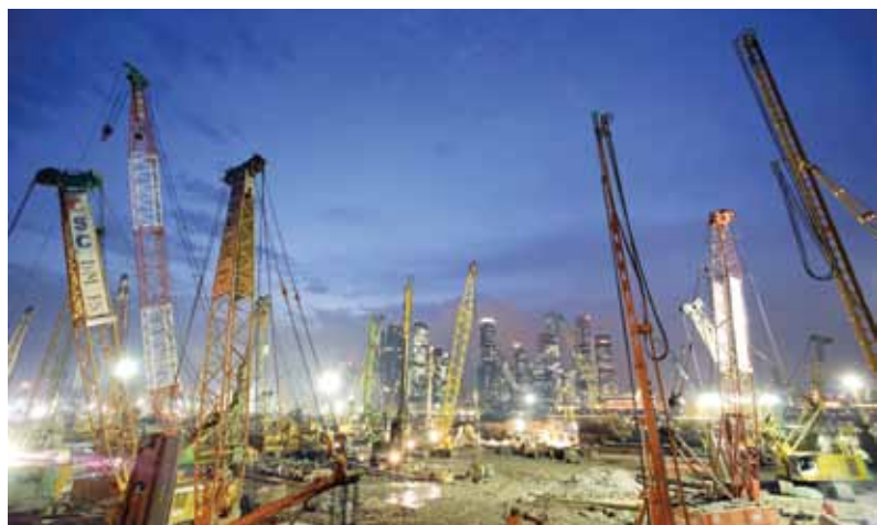
Figure 2: The site was quickly engulfed by a sea of cranes in order to achieve the very aggressive construction schedule. Courtesy of Arup.
