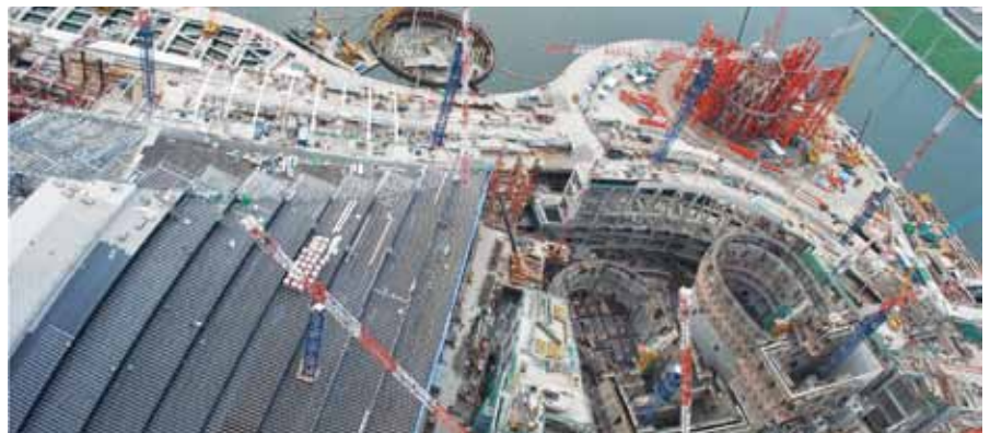
Figure 7: View from atop the hotel looking down upon the waveform casino roof and the dual theatre buildings still under construction at the time of this photo. The ArtScience Museum's hyperbolic diagrid is seen under construction at top right. Courtesy of Arup.
