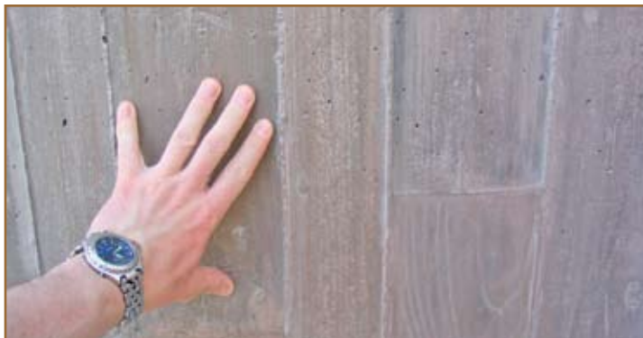
The use of Self-Consolidating Concrete (SCC) resulted in a superior finish and cost savings due to the significant reduction in the need for cosmetic repairs typically necessary when using traditional cast-in-place concrete.
