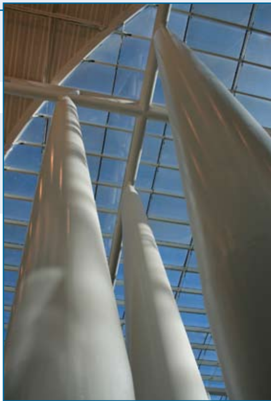
Slender roof columns taper at each end to a single pin connection.
