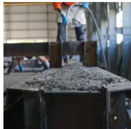
Figure 7: EFC geopolymer concrete being vibrated into the beam molds, at Precast Concrete Pty Ltd factory, Brisbane.
