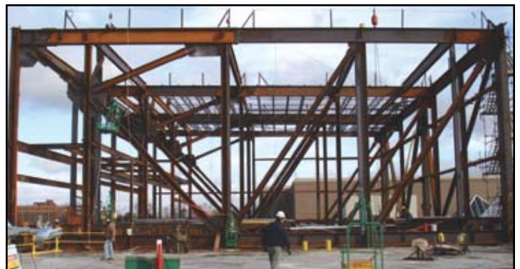
100-foot-long trusses run east-west over the existing mall roof. Courtesy of Douglas Platt, McLaren Engineering Group.
