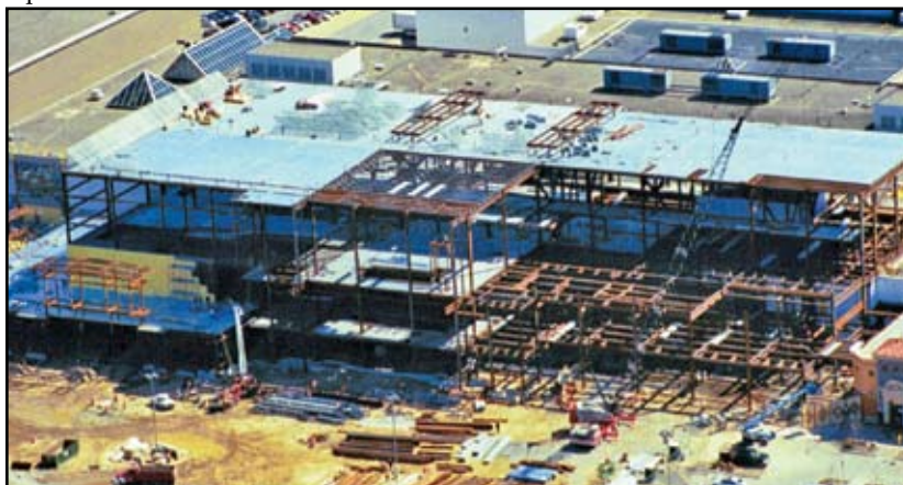
Aerial view shows structural steel being assembled during the expansion of the Colonie Center Mall in Albany, N.Y. Courtesy of Turner Construction Co.
