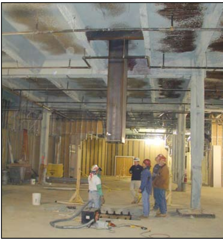
Workers thread super column through existing building onto new base plate and footing. Courtesy of Turner Construction Co.
