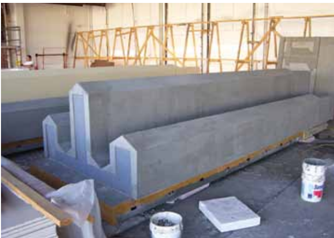
Figure 2: Pilaster element during the finishing process. Courtesy of Chicago Panel and Truss.
