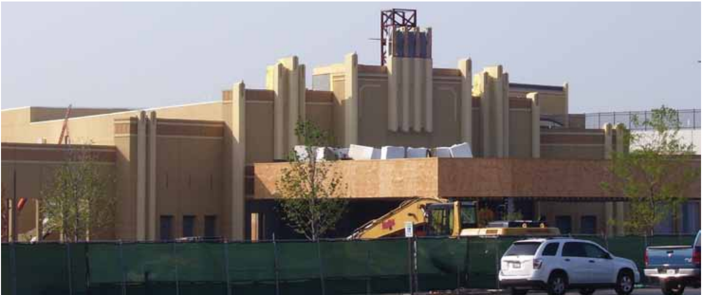
Figure 4: Main entry of pavilion after completion of prefab wall panel installation. Courtesy of Chicago Panel and Truss.
