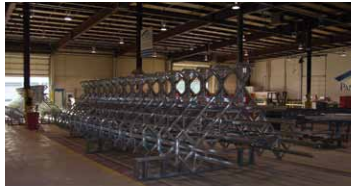
Corner feature of parking structure ready for sheathing and finish. Courtesy of Chicago Panel and Truss.
