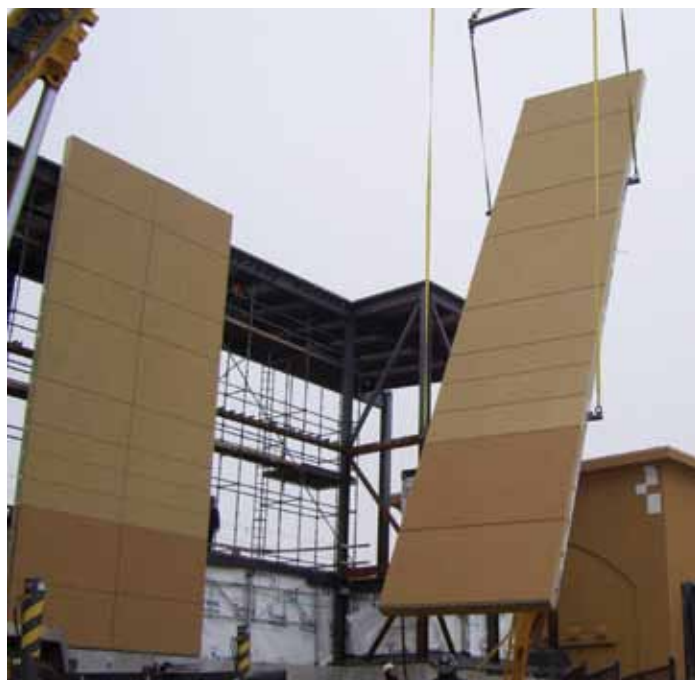
Figure 1: 45-foot tall wall panel being hoisted into place. Courtesy of Salamone Builders.
