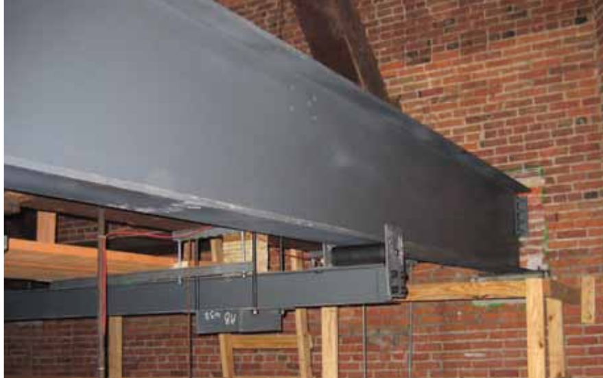
Detail of the framing and roller supports to guide W24 girders into their bearing pockets.
