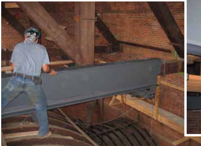
New steel was inserted in the attic to support the historic timber roof trusses.
