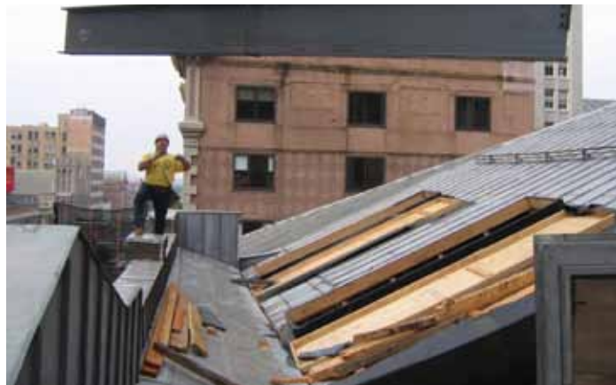
Rooftop view of steel being inserted into the Academy of Music attic.
