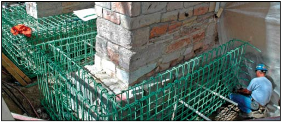
The sandstone piers and their foundations were reinforced to prevent failure in an earthquake.
