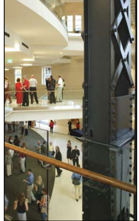
Existing Built-Up Columns To AESS Standards Restored. Courtesy of Ron Pollard, Photographer.
