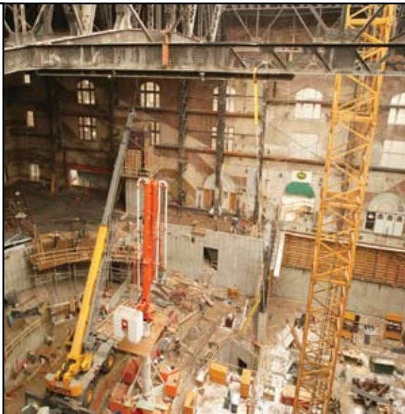
Concurrent Demolition, Foundation Underpinning, Structural Bracing And New Construction. Courtesy of Martin/Martin.
