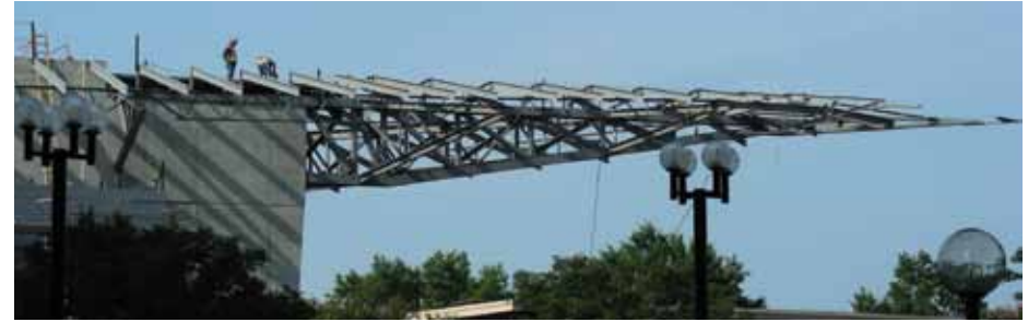
Courtesy of Bing Thom Architects. Fast + Epp was an Award Winner for the Arena Stage at the Mead Center for American Theater project in the 2011 NCSEA Annual Excellence in Structural Engineering Awards Program (Category – New Buildings over $100 Million)
