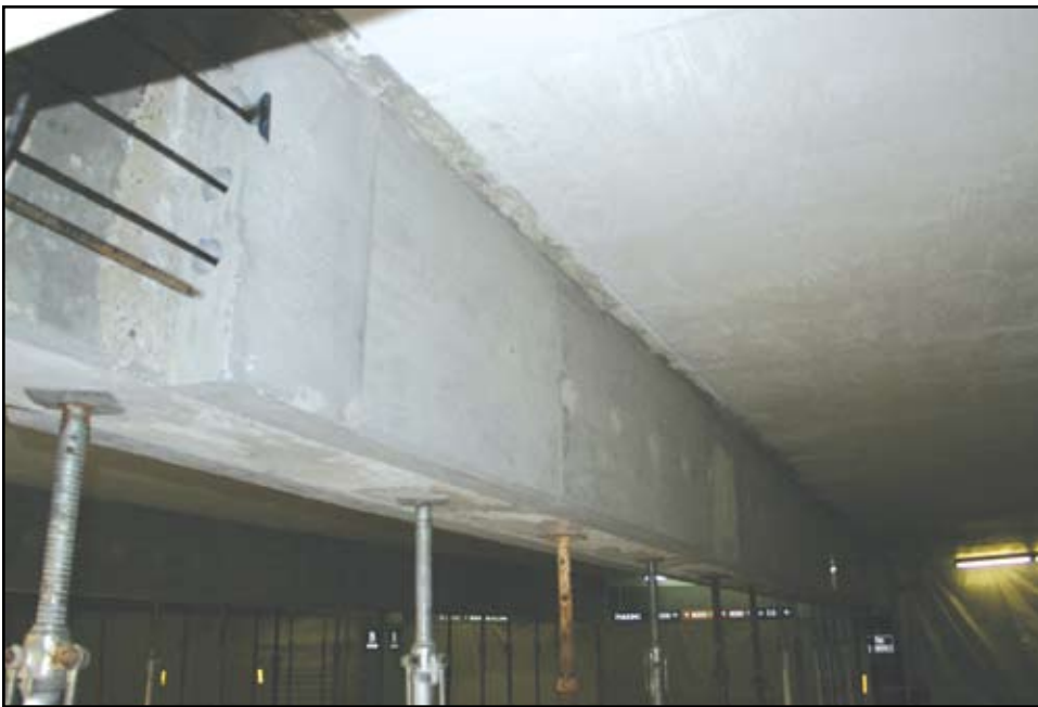
Final beam – pumped, cured and stripped – prior to stress of the cables and pouring of the stress block at the end.
