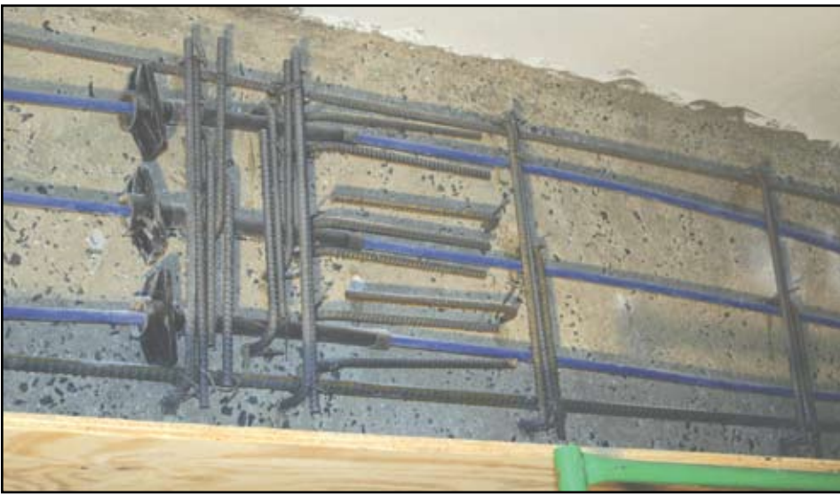
Close up of PT cable anchors and rebar prior to formwork installation.
