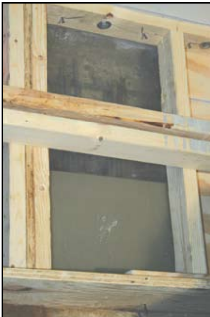
Pumping in progress with SCC filling up the plexiglass viewing window. The window was built into the formwork at the end anchors.
