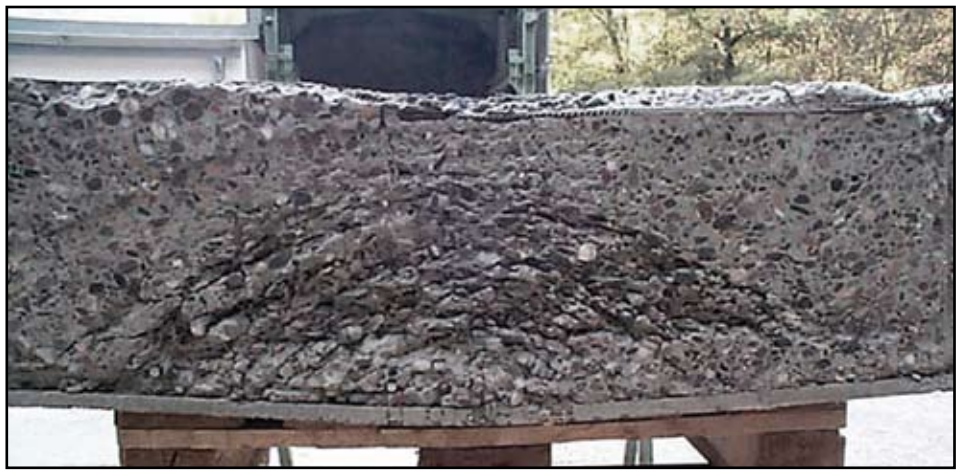
The top 12 inches of this slab is standard reinforced concrete, subjected to blast loading on the upper surface. Transferred blast energy caused a spall of approximately 75% of the concrete thickness off the bottom of the standard concrete portion, clearly visible as a dome-shaped crack. The 0.6-inch MRC fragmentation-protection layer at the bottom successfully contained this spall.
