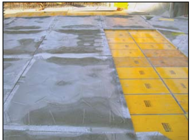
Precast MRC panels are placed over a basement high-security data center. They will be overlaid with a deck of standard concrete that will form the floor of the building's main lobby.
