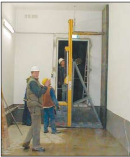
An MRC panel is installed in a European broadcasting center. A publicly accessible parking garage abuts the right wall, creating a vulnerability, but the MRC panels provides both blast absorption and fragmentation protection. The precast panels were lowered into the corridor through a slot cut in the ceiling.
