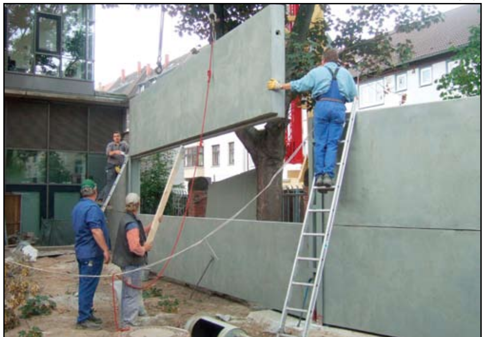
Precast MRC panels are attached to simple steel post supports to form a free-standing blast wall protecting a vulnerable community center.
