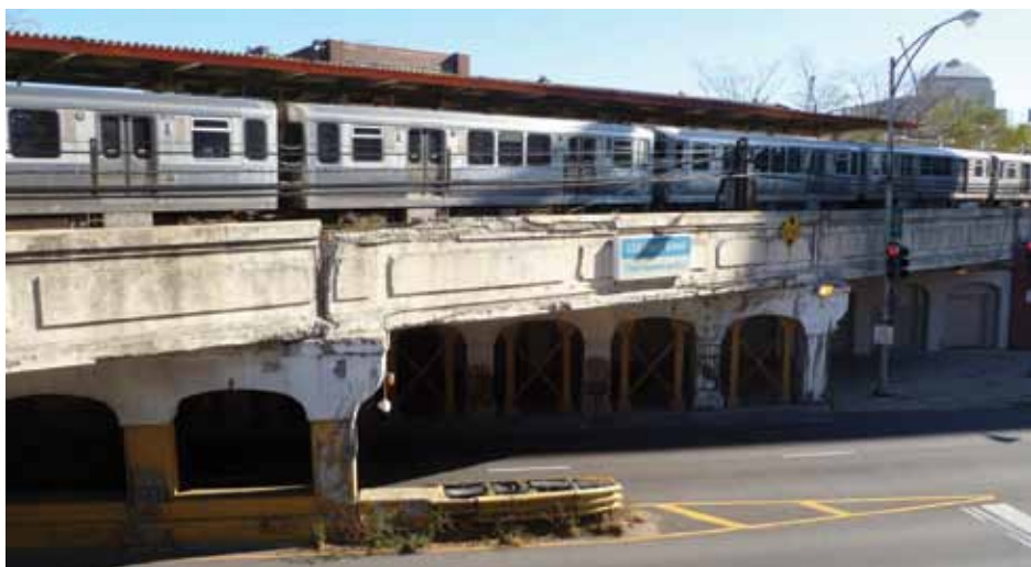
Figure 1: Corrosion-damaged concrete piles in Chicago being assisted with steel trusses.
