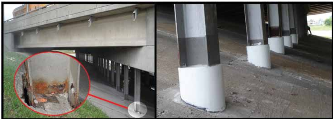
Figure 4: The I-70/I-270 interchanges in St. Louis, MO where 49 corroded bridge piling were recently repaired with FRP laminates.
