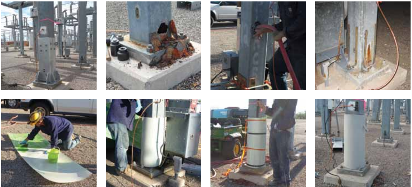
Figure 3: Repair of steel poles at TEP substations: original repair concept; corroded pole; filling the pole with grout; reinforcing steel welded to base plate; applying epoxy to the laminate, wrapping it around the pole and holding it with straps while grout is placed; finished and painted jacket.
