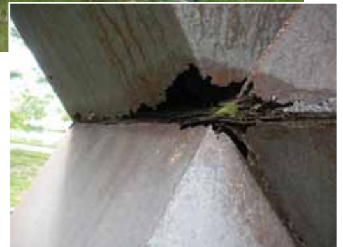
Right: Corroded Steel at the Center of the Sculpture.
