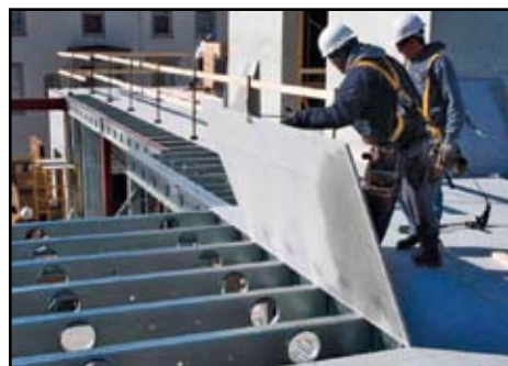
Figure 3: Cement-based flooring: proprietary product from USG called Fortacrete. Courtesy of USG.
