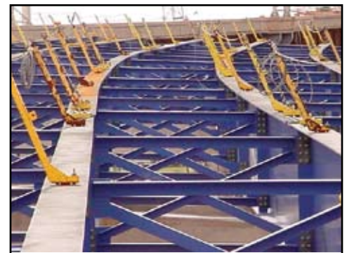
The Marquette Interchange in Milwaukee is an example where performance based specifications resulted in a two coat system replacing the traditional three coat bridge coatings. Courtesy of Tony Holzinger.
