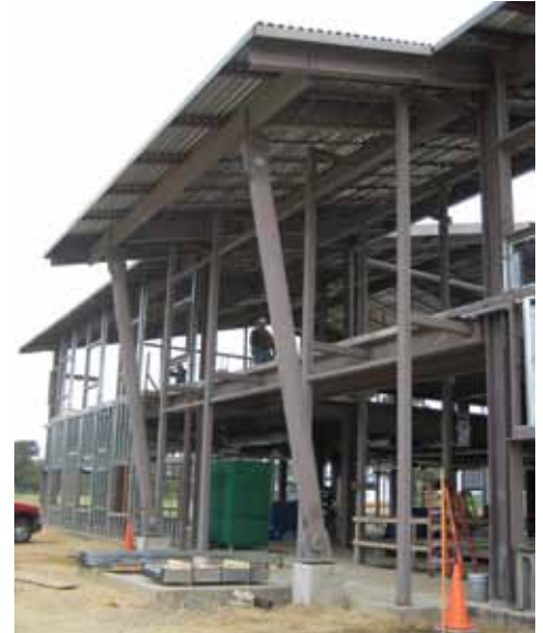
Figure 1: Cast Connex® Universal Pin Connectors™ used in the Air National Guard Operations and Training Facility, New Jersey. Courtesy of Carlos de Oliveira, Cast Connex Corporation.
