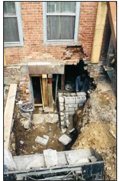
Restoration of an 18 th century exterior masonry wall. Jack under lintel – wall is rebuilt on concrete footing. Courtesy of Mark Mendel.
