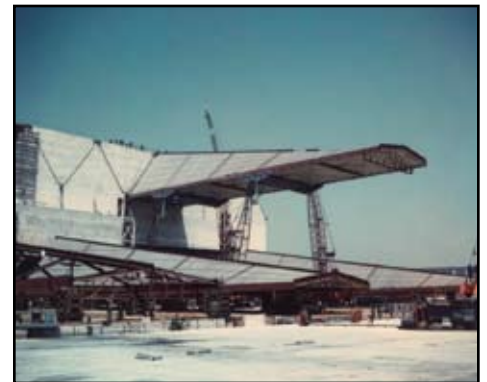
American Airlines Hanger under construction. Los Angeles and San Francisco, CA. Courtesy of C.H. Thornton and Thornton-Tomasetti Group.
