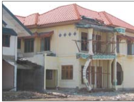
Column failure due to debris impact.
