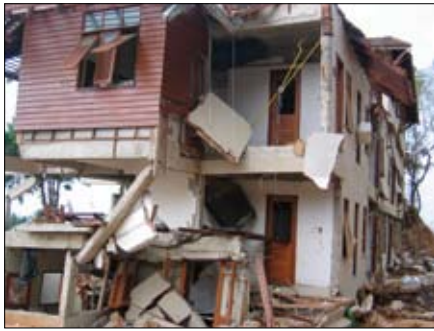
Severe structural damage.
