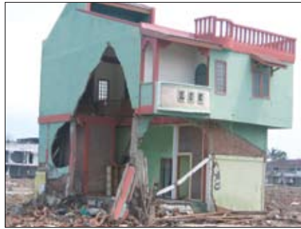
Punching failure of infill walls.
