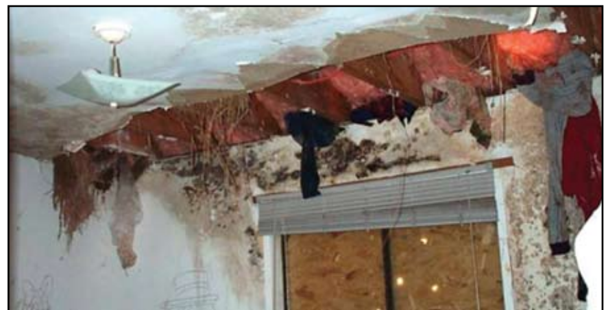
Figure 2: Water is driven in by the wind causing further damage and leading to mould growth.
