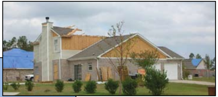
Figure 1: Wind-storm causes extensive damage to light-frame houses in the Greater Toronto Area.
