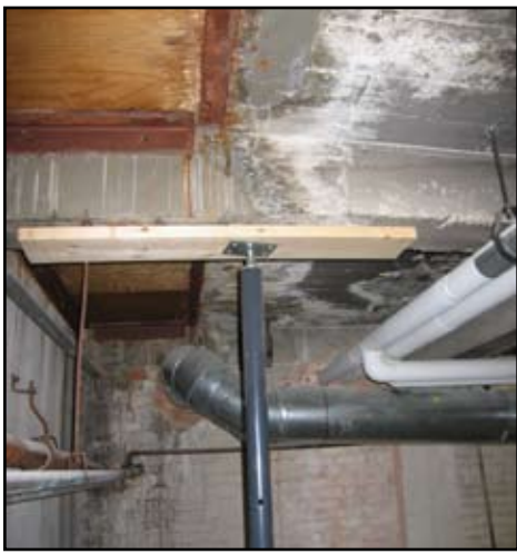
Figure 3: Concrete beams and slabs forming the vault cover. Note the shored beam and leaching on the slab underside caused by moisture migrating from the top.
