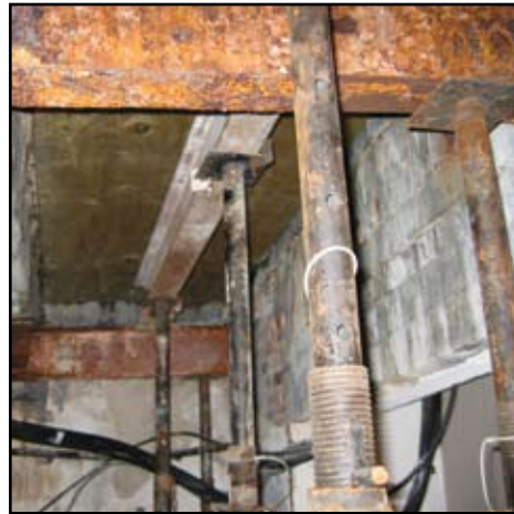
Figure 4: Shoring of a deteriorated vault structure.
