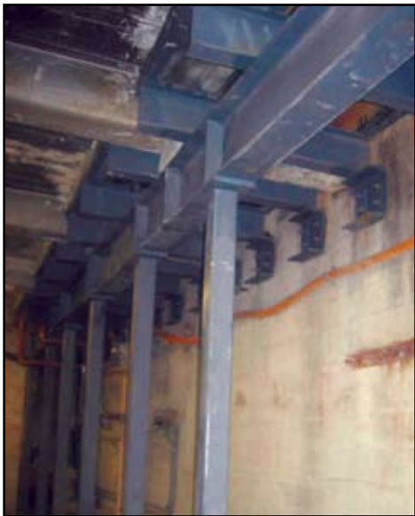
Figure 6: New steel structural support for partial replacement of a vault cover. Note that the original structure consists of concrete beams and slabs.
