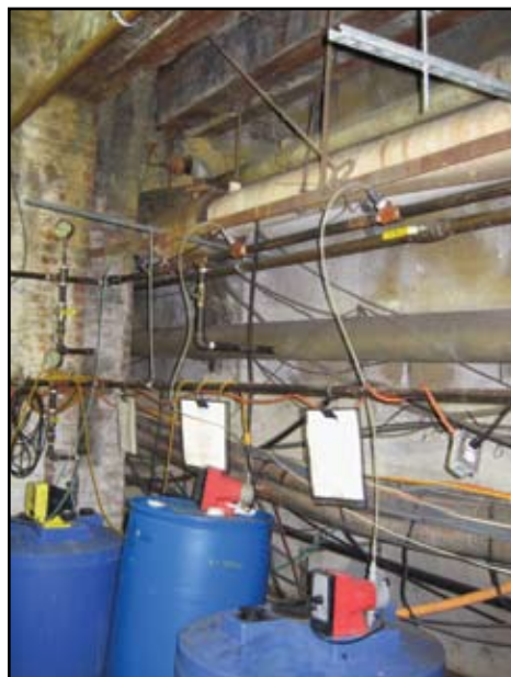
Figure 7: Vault space congested with utility lines.
