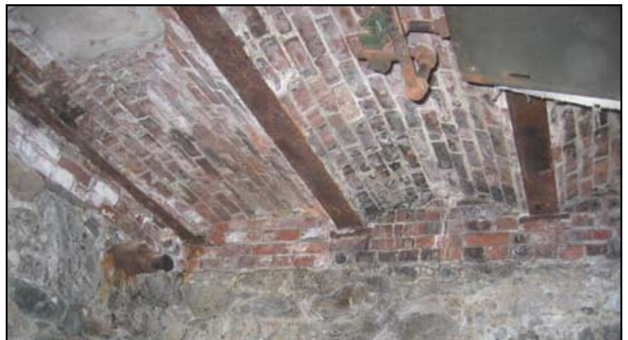
Figure 2: Segmental masonry brick arches supported by steel beams and stone masonry walls.
