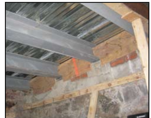
Figure 5: Support for new cover vault consisting of metal deck and steel framing.
