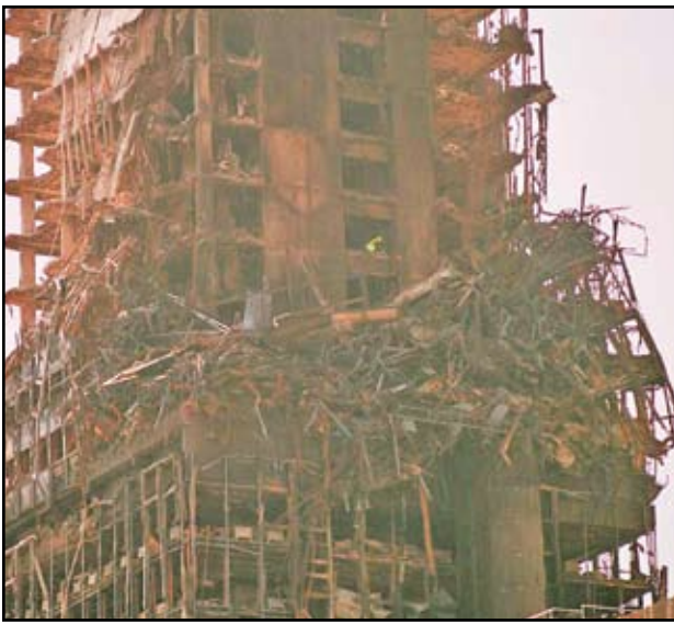
Windsor Building in Madrid, Spain after fire burnout – a portion of the building that experienced partial collapse. Courtesy of Vicent Pons.
