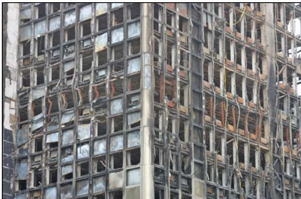
Windsor Building in Madrid, Spain after fire burnout – a portion of the building that withstood the fire. Courtesy of Ramon Gilsanz.
