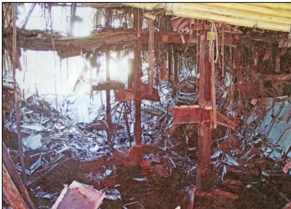
Figure 1: Internal Collapse Area in WTC 5 (FEMA, 2002, p. 4-18).
