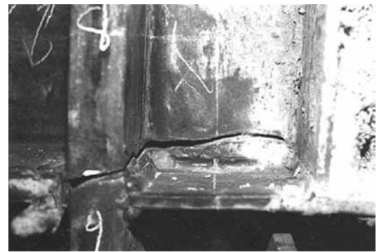
Figure 4: Fracturing of a W14 column at the welded beam-to-column connection. Courtesy of the SAC Joint Venture.
