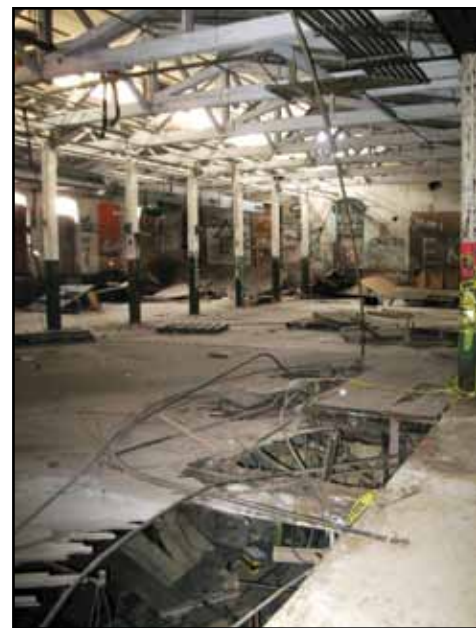
Collapsed 1 st Floor Framing over Basement.
