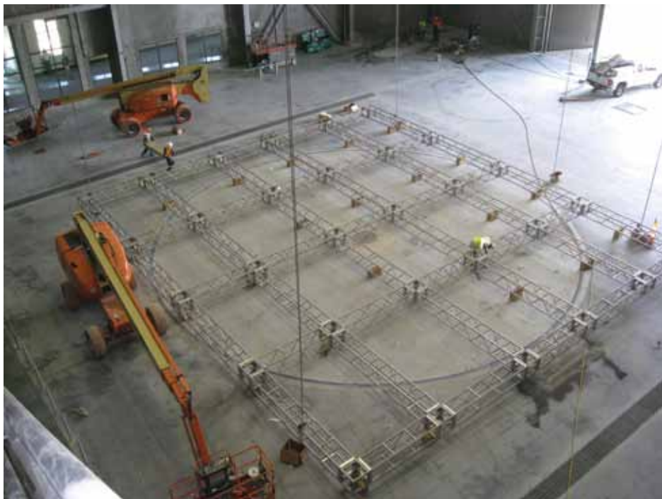
The aluminum deluge truss rig being assembled on the test chamber floor just above the turntable. Courtesy WALTER P MOORE.
