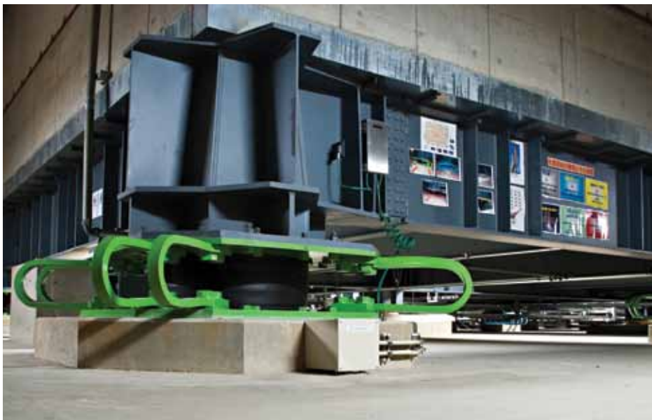
Overall view of the isolation basement of the Ishinomaki Red Cross Hospital. The isolation system comprises about 100 natural rubber bearings and U-shaped steel dampers. (Photo: SIE, Inc.)
