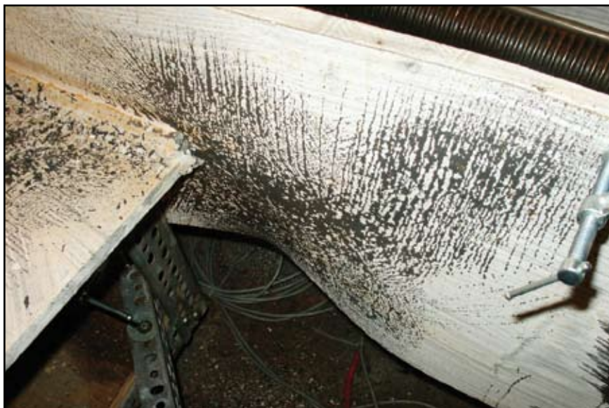
Figure 1: Extensive Yielding in Beam and Column.
