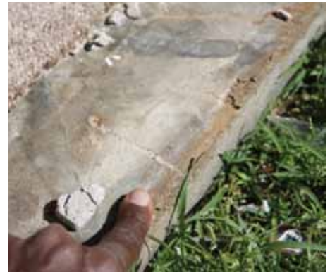
Figure 3: Evidence of cut nail at sill plate.
