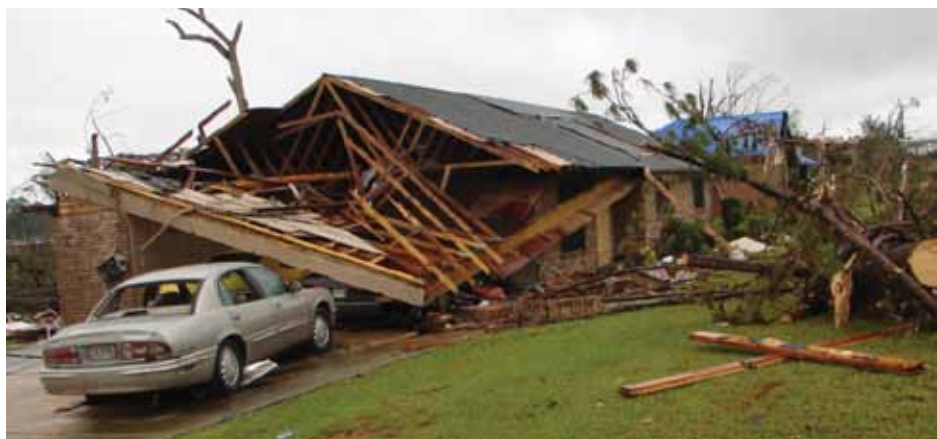
Figure 2: Carport column uplift failure.
