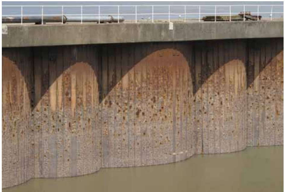
Steel piles form the cylindrical cofferdams. Between the cofferdams are additional arcs of steel piles, making much of the cofferdam piles inaccessible.
