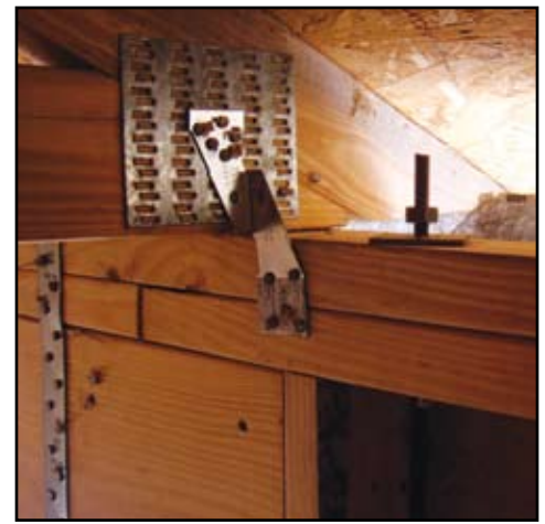
Figure 7: What was once a nut tightly secured to the bearing plate now has a gap, as wood shrinkage and dead load compression occur throughout the structure.
