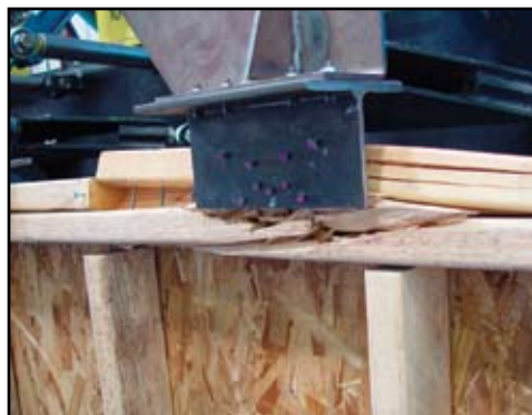
Figure 5: With rods centered in the wall and sheathing on opposite side of wall, cross-grain tension failure occurs as top plate bends upward. Mechanical reinforcement is needed.
