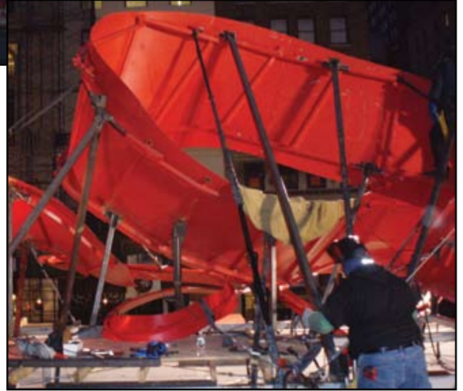
Fabricating the red ribbon bow, which was 12 feet high, 50 feet long, weighed 3 tons and made of 10-gauge steel. Courtesy of McLaren Engineering Group.
