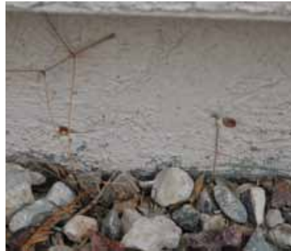
Figure 1: Rust Marks of Burned off Anchor Nails.
