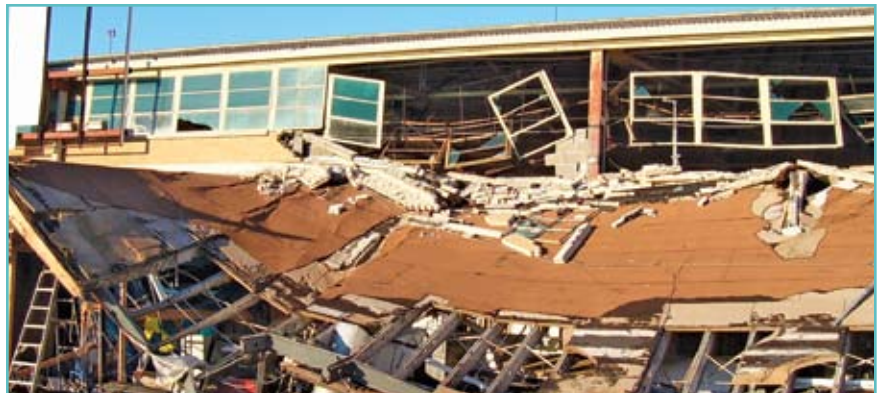
Partial Collapse of the Wendell Hanger, Lakefront Airport, New Orleans, LA., Courtesy of Ed Huston, Smith & Huston, Inc., All Rights Reserved.
