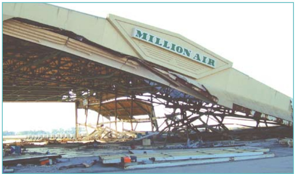
Partial Collapse of the Million Air Hanger, Lakefront Airport, New Orleans, LA., Courtesy of Ed Huston, Smith & Huston, Inc., All Rights Reserved.
