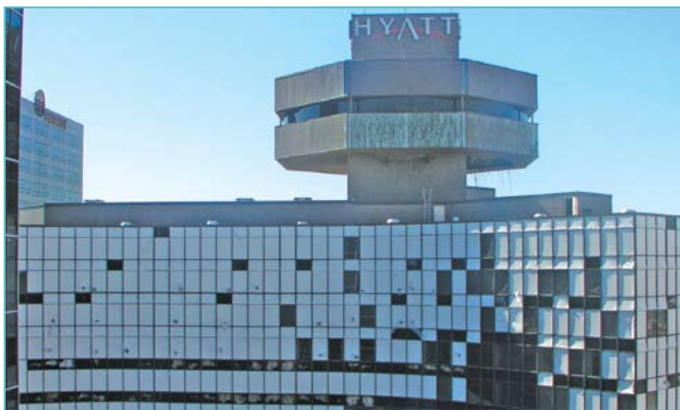
Wind-borne debris glazing damage to hotel in New Orleans, LA. Courtesy of Ed Huston, Smith & Huston, Inc., All Rights Reserved.
