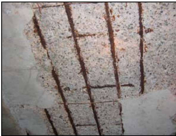
Figure 1: Deterioration of concrete due to rebar corrosion.
