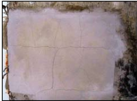
Figure 5: Shrinkage cracking of patch due to lack of proper curing.
