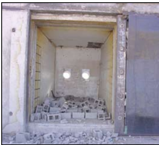
Figure 7: Un-retrofitted and CFRP retrofitted URM walls after the blast test.
