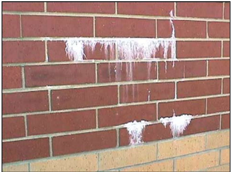
Figure 5: Lime runs in brick wall.
