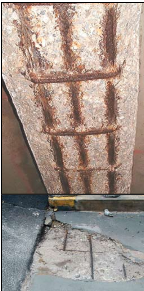
Figure 1: Deterioration of Concrete Due to Rebar Corrosion.
