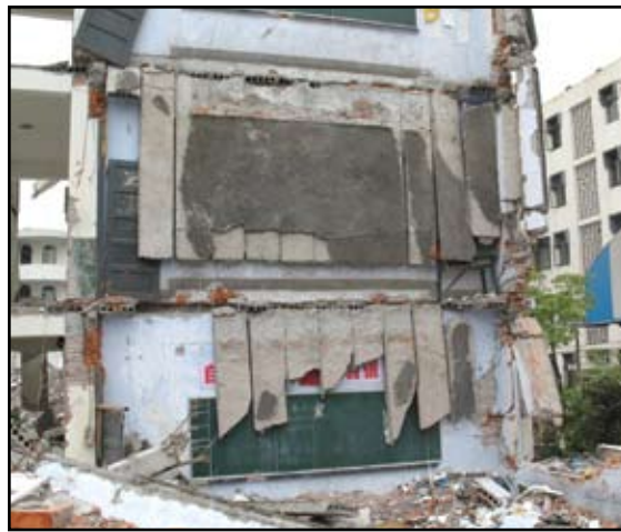
Figure 1: URM wall and RC floor plank collapse, Juyuan Middle School.
