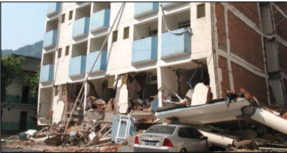
Figure 2: Soft-story collapse, Hanwang Hospital.
