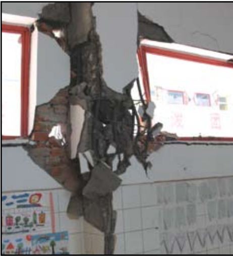
Figure 3: Captive column failure, Hanwang High School.
