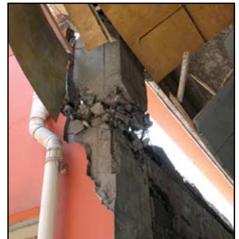
Figure 4: Column flexural damage, Mianzhu Experimental School.
