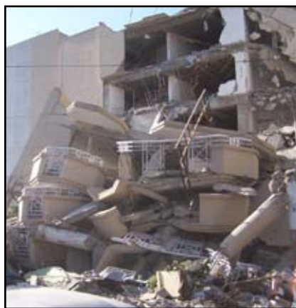
Figure 1: Poor Structural Performance of MICF Buildings During Earthquake. Courtesy of A. Nisar (MMI Engineering EERI).
