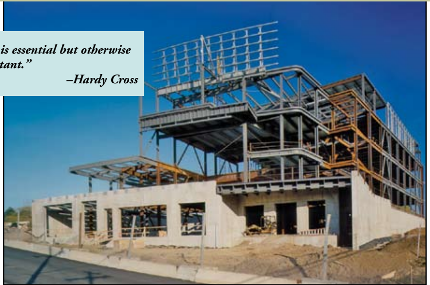
Steel framed laboratory building; University at Albany Center for Excellence in Cancer Genomics.
