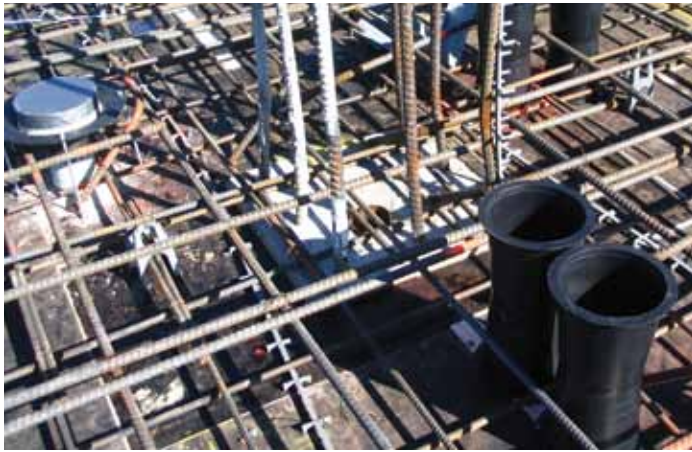
Figure 3: Unanticipated Slab Openings.
