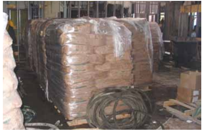
Figure 4: Unanticipated Construction Loads.
