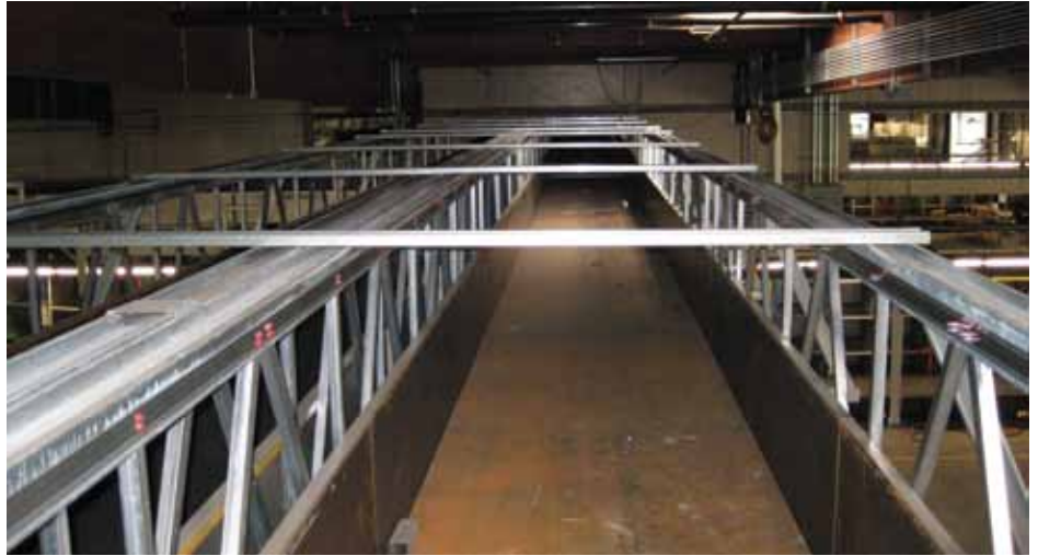
Figure 4: Double wide conveyor with lateral braces.
