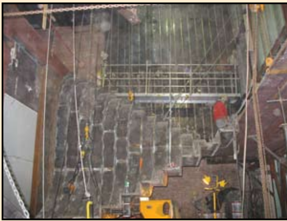
Construction: Looking south at the second floor on left and upper mezzanine and cantilever on the right.
