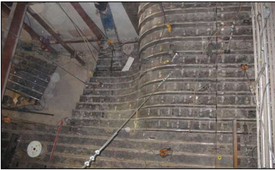
Figure 5: View from above - construction work proceeded from the second floor, at top of photo toward the north (at left).
