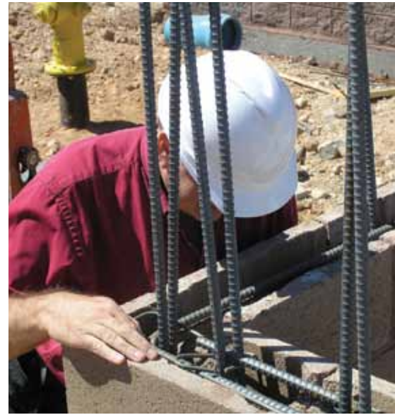
Inspection of reinforcement location and cleanliness of cells prior to grouting. Courtesy of Masonry Institute of America.
