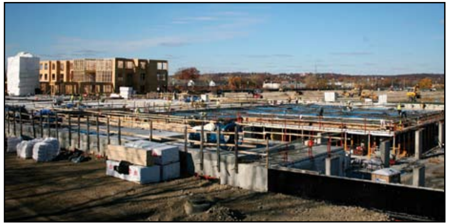
The photo above shows the sequence of construction from right to left beginning with the column spacing for parking, the post-tensioning being placed, a poured slab and finally the wood framing being erected. Courtesy of Plumb House Inc.
